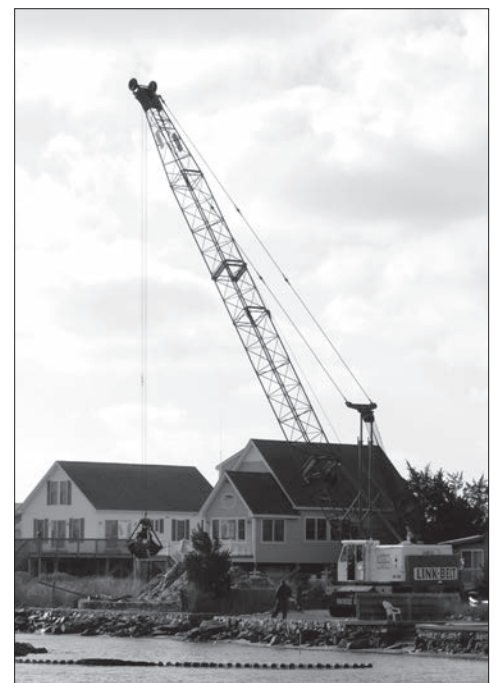
A clamshell bucket dredges the Breach Drive spur of the Weekapaug breachway.
